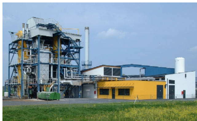
Biomass steam gasification plant at Güssing, Austria. (Courtesy R. Rauch)
