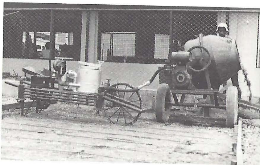
Manila, Philippines, 1982. A charcoal-fueled portable gas generator that can be wheeled to different sites to power small equipment such as the concrete mixer shown here. (GEMCOR, Manila)
