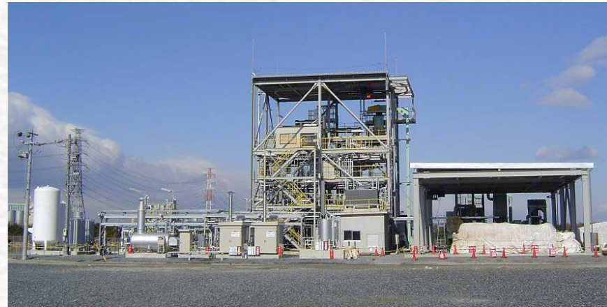
Overview of 2t /day test plant
