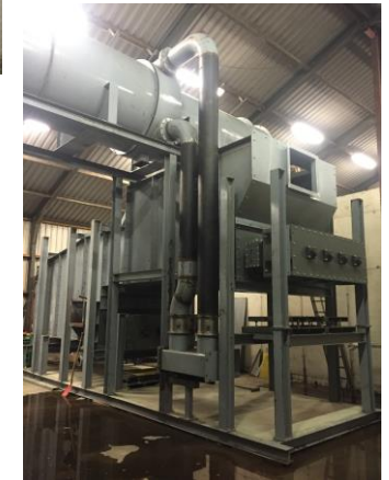
Swine manure gasifier
