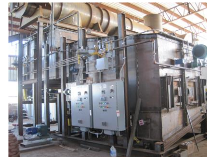
Digestate (cow manure) gasifier
