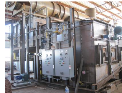
Digestate (cow manure) gasifier
