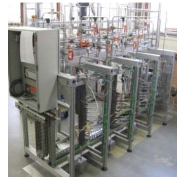
Further gas cleaning
