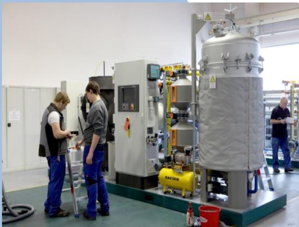
50 kWel plant from Burkhardt GmbH
