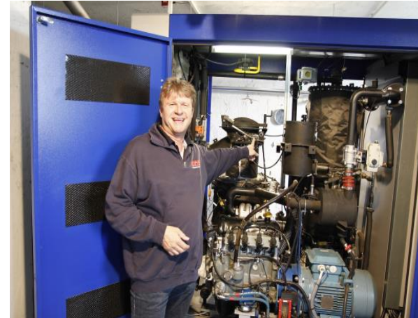
9kWel plant from Spanner Re 2 GmbH
