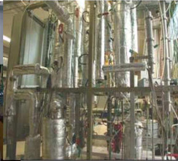
OLGA Gas cleaning
