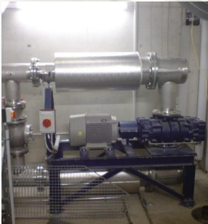
Root's compressor located next to the CHP
