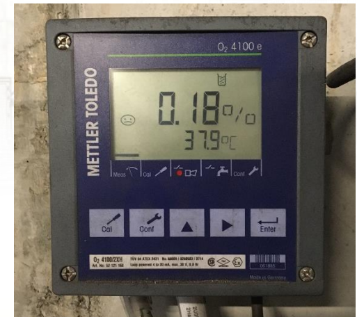
display for redundant analysis module
