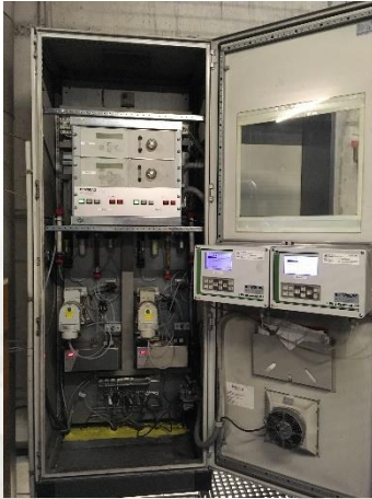
blower, dryer, filter
