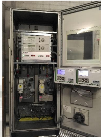
blower, dryer, filter
