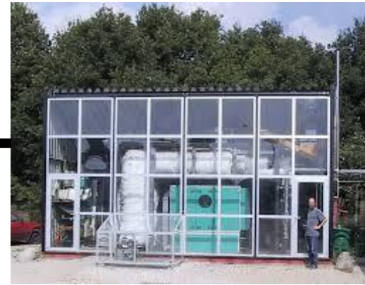
Viking Gasifier (Danish Technical University)
