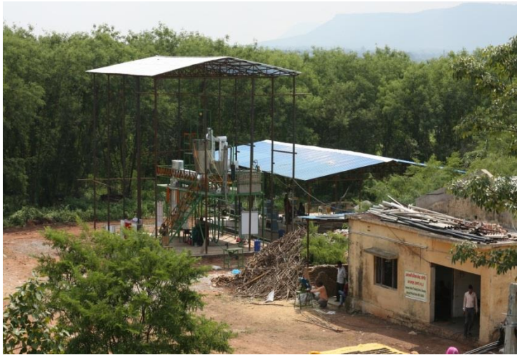
Biomass Gasifier for electricity production
