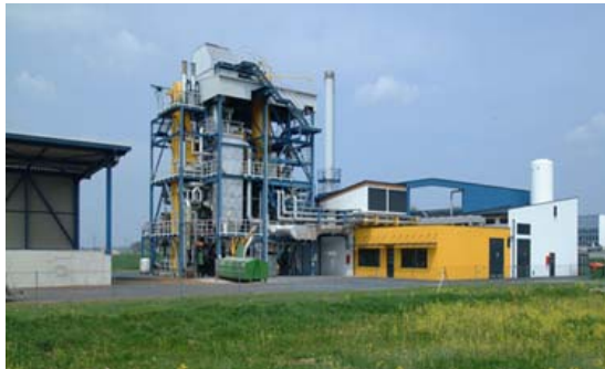
8 MW demonstration plant Güssing
