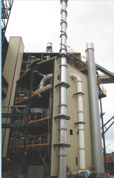
Figure 1 Gasifier general view
