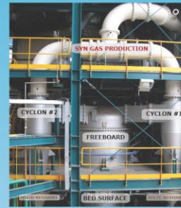
Figure 2 Gasifier, cyclones and syngas outlet duct
