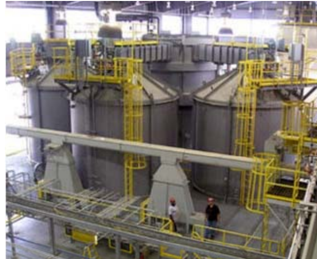
Gasifiers and metering bins at USC plant
