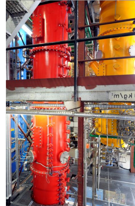
200 kW th (not el. heated)
