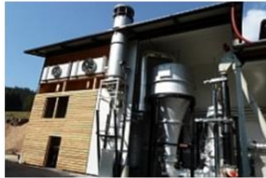
Wood gas power plant
