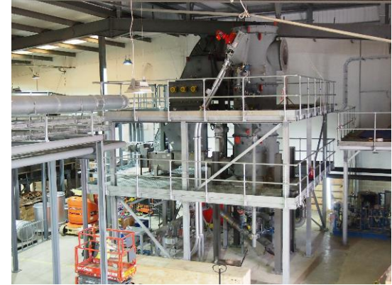
Demonstration plant gasifier
