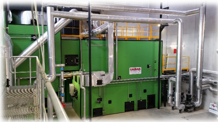
Hot water boiler
