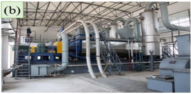
The gasification & combustion sections
