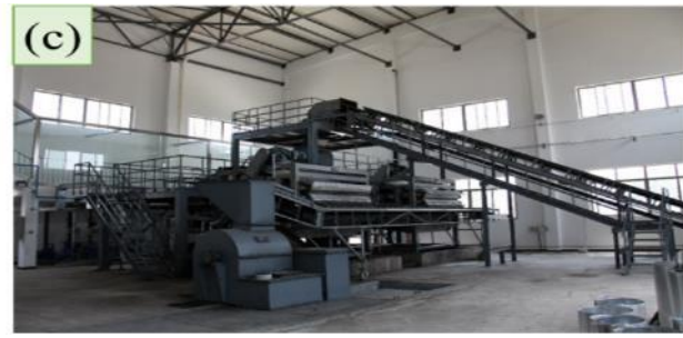
The crushing & drying sections
