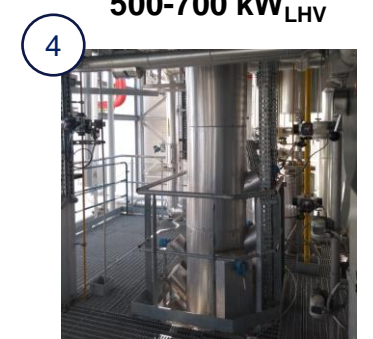
Reactor installed on the GAYA platform (~ 400-600 kW LHV SNG)
