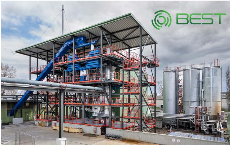
1 MW DFB gasifier
