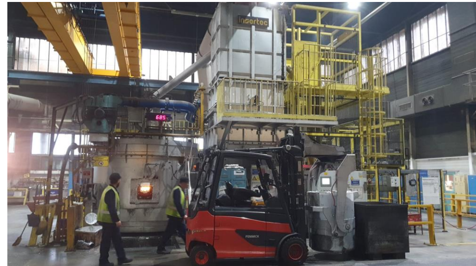
Insertec 1 Stellantis furnace
