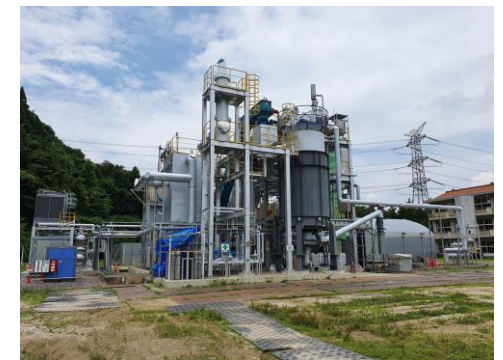
Charmey Regawatt CHP plant – (CH)
