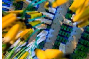
Grid Computing Centre Karlsruhe (GridKa)
