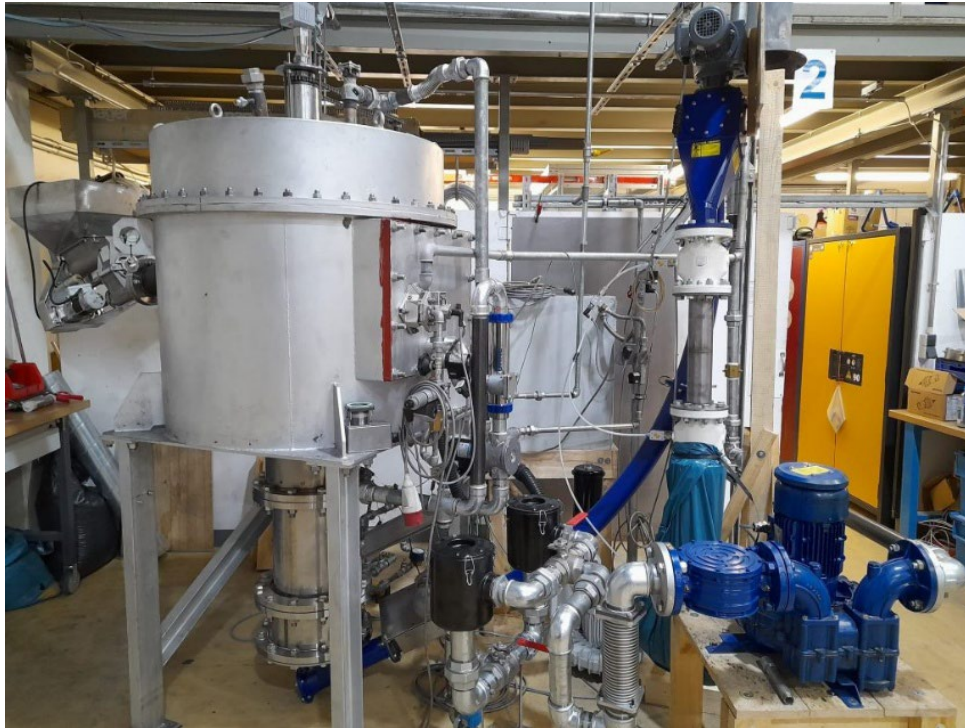
Figure 7: Picture of the BtX Energy test facility
